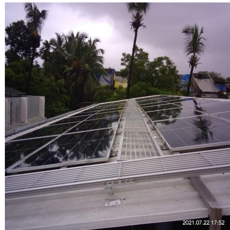
Tejomayee II Solar Panel Installation completed at IWSAHQ, Nov. 2021.
