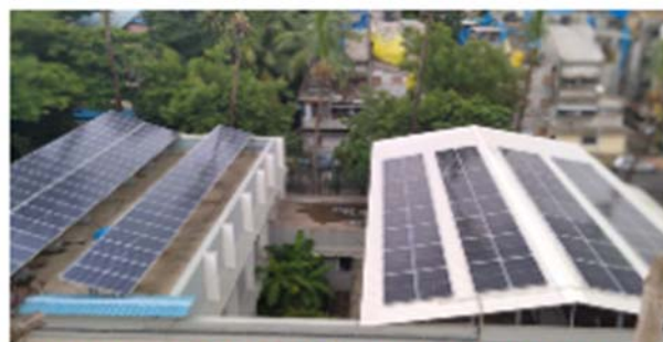
Solar System for electricity 21 KWp + 25 KWp
